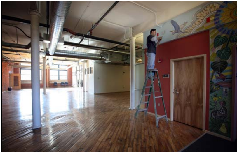
Rogelio Villalta puts finishing touches on one of the walls leading to a common area at Union Crossing, a housing development at the old Southwick Clothing site on Island Street in Lawrence.
